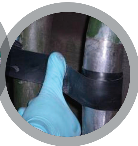
Oil Leak Repair
